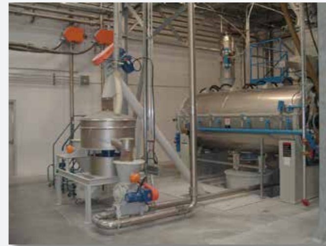
COOLER DISCHARGE AND SIFTING SYSTEM
