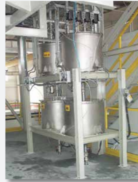
OIL WEIGHING SYSTEM
